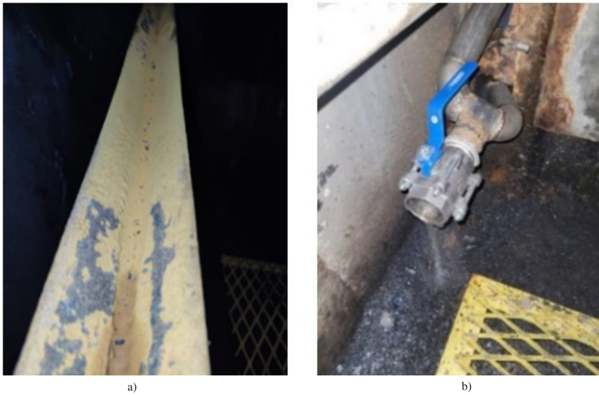
Figure 4. (a) Channel for water collection and (b) opening valve.
